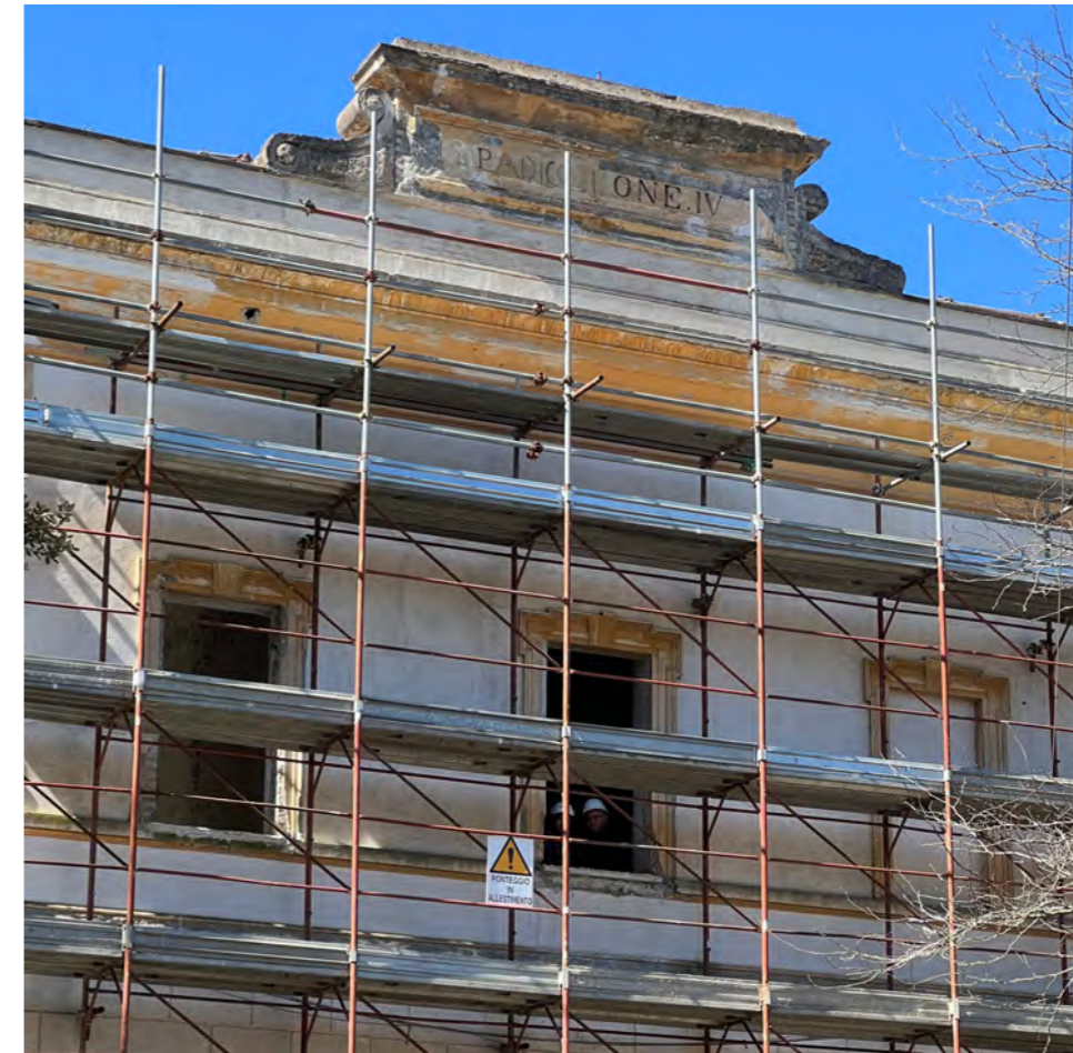
Former Santa Maria della Pietà Psychiatric Hospital, Rome. Renovation to re-functionalize the complex for the neighbourhood
