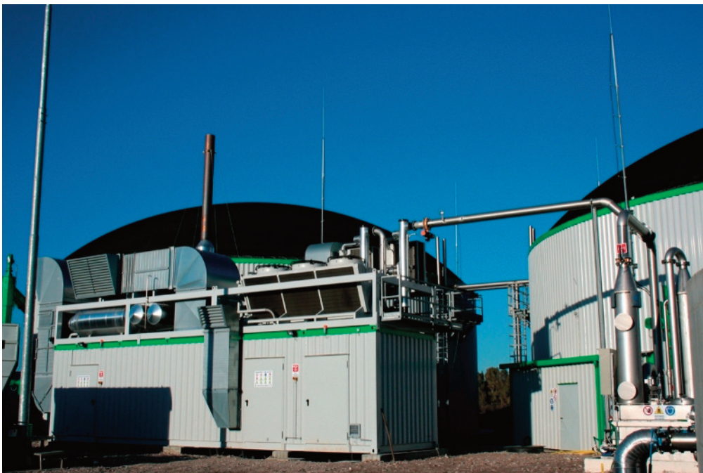
Figure 7. Biogas Production Plant
